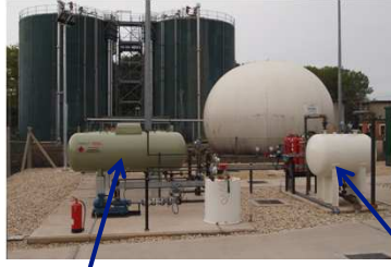
Propane Storage tanks
